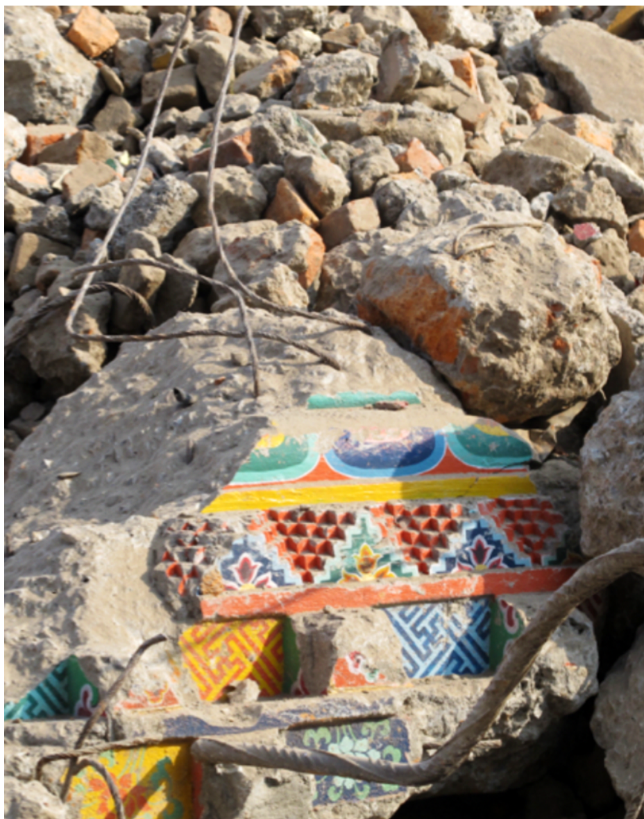
Even though this monastery was well-constructed with concrete, due to its location it suffered severe earthquake damage
