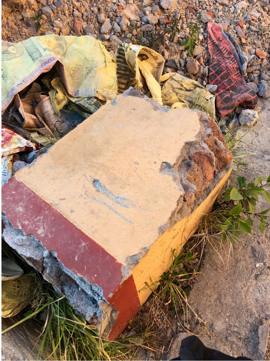
Pillar of monastery that was built on a mountaintop. Most of this monastery was damaged so severely it had to be removed and completely rebuilt.
