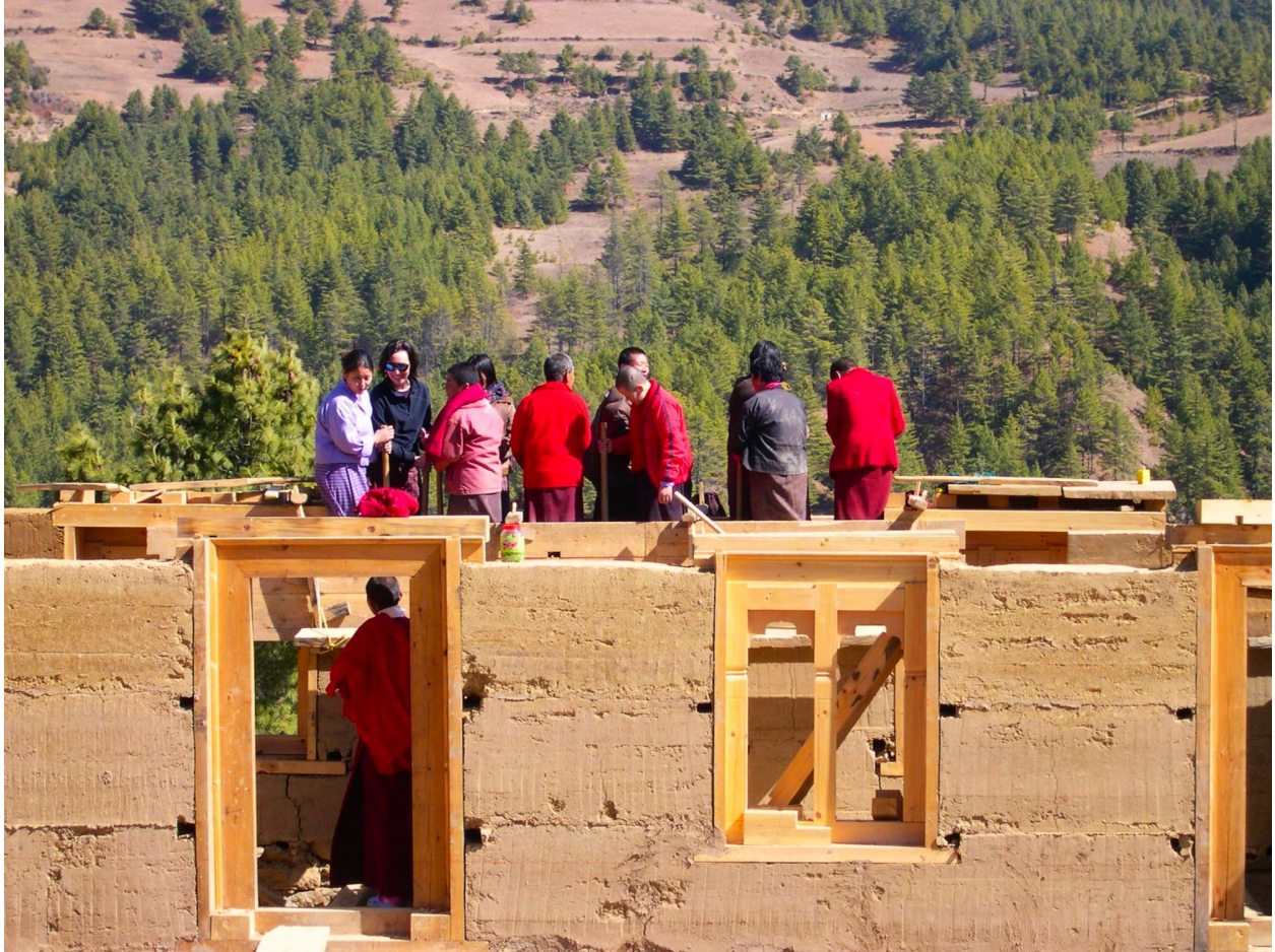
Nuns building their own monastery in a traditional, pounded-earth technique. Some people believe that traditional structures are stronger during earthquakes than concrete buildings.
